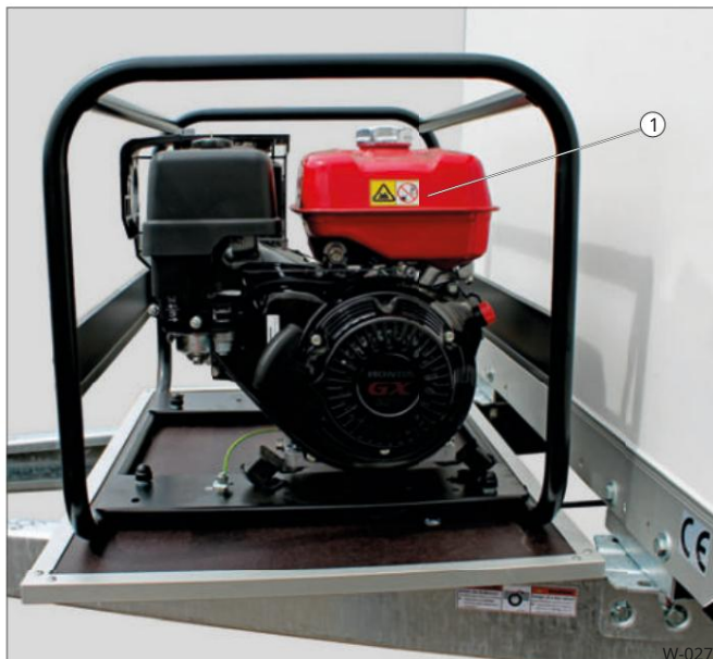
Sl. 28 Generator snage 1 spremnik goriva
